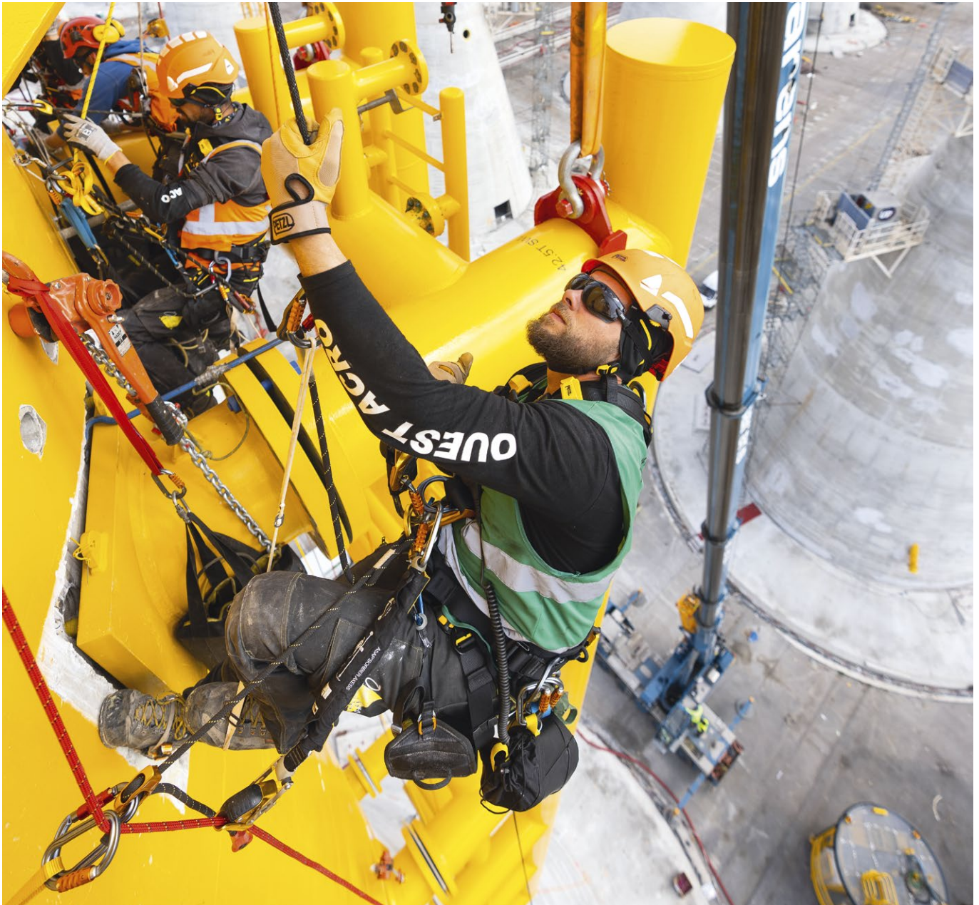
Construction of gravity-based foundations for an offshore wind farm, Le Havre, France © 2022 Petzl Distribution - Vuedici.org - Ouest Acro - Bouygues travaux publics - Fécamp offshore wind farm
